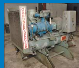
75 HP Gardner Denver Electric Screw Air Compressor
