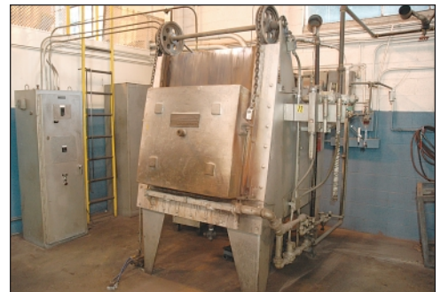
Lindberg Type 11-R0-243618-20A Natural Gas Fired Furnace
