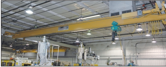
(2) 3 Ton X 45' Approx. Span CMH P&H Single Girder Bottom Running Overhead Bridge Cranes
