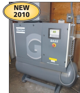
30 HP Atlas Copco Model GA22 Rotary Screw Horizontal Tank Air Compressor
