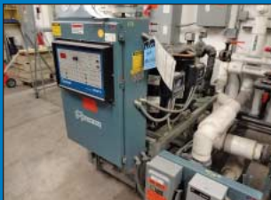
(2) 20 Ton Advanced Engineering Water Condensed Central Chillers
