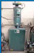
Unidyne Central Vacuum Pump System with (2) 5 HP Vacuum Pumps
