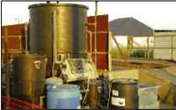
TRIANGLE EQUIPMENT OILY WATER TREATMENT SYSTEM
