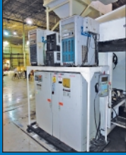
Close Up View Power Supplies and Control In Welding Cell
