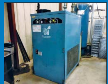
(2) Arrow Model 3517-4 Refrigerant Air Dryers
