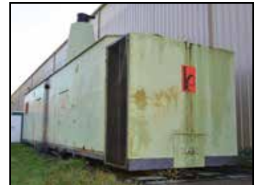
GENERAL MOTORS MP45A Generator
