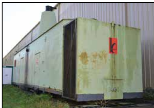
GENERAL MOTORS MP45A Generator
