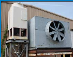
Cooling Tower System Including Cooling Tower Cells
