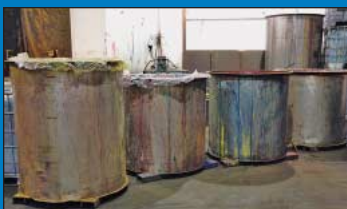
Partial View Stainless Steel Tanks
