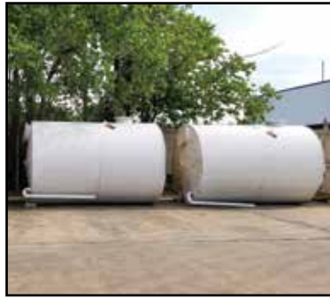
(3) 4,200-Gallon Storage Tanks
