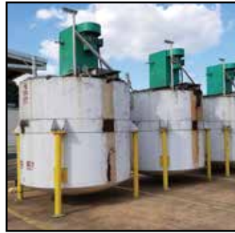
(4) TSM 2,500-Gallon Let Down Tanks w/SCHOLD Agitators
