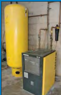
Close Up View Dryer and Tank
