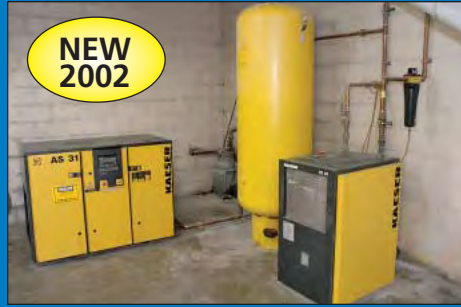
Overall View Air Compressor System Including 25 HP Kaeser Model AS31 Compressor, Dryer and Tank
