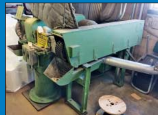
DE Sander / Buffer w/ Dustkop Dust Collector
