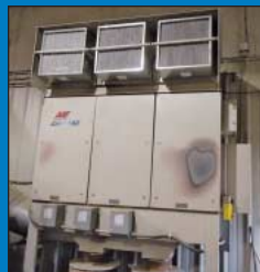
10 HP and 5 HP AAF American Air Filter Dust Collectors
