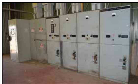
GENERAL ELECTRIC 7700 Line Motor Control Center
